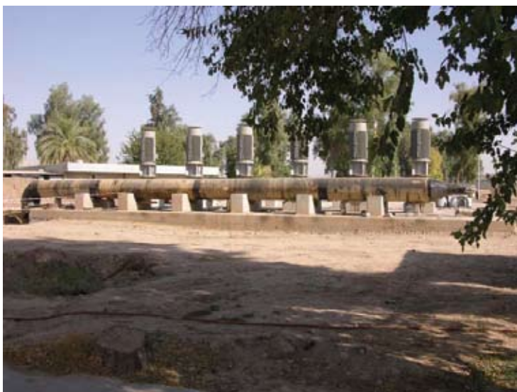
Dibbis Pump Station.
