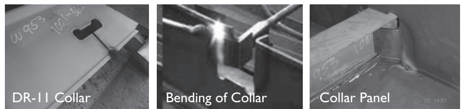
Figure 5. Photographs showing a bendable tab design being employed for construction of the hydrostatic tests panels at Northrop Grumman Ship Systems.
