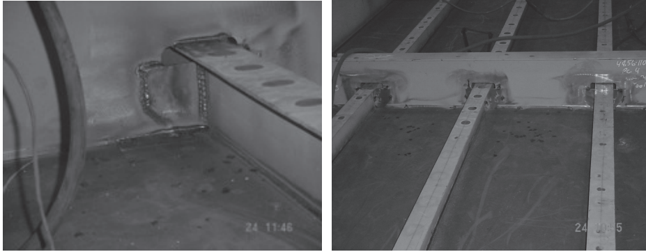
Figure 1. Photographs showing collar details and structure for a typical arrangement used for ship construction.
