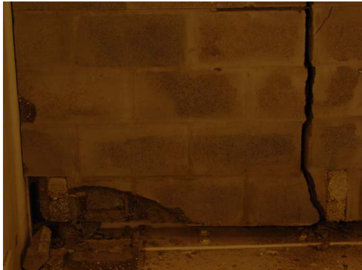
Fig. 3.44. Bottom support failure of Wall 3 in Detonation 2
