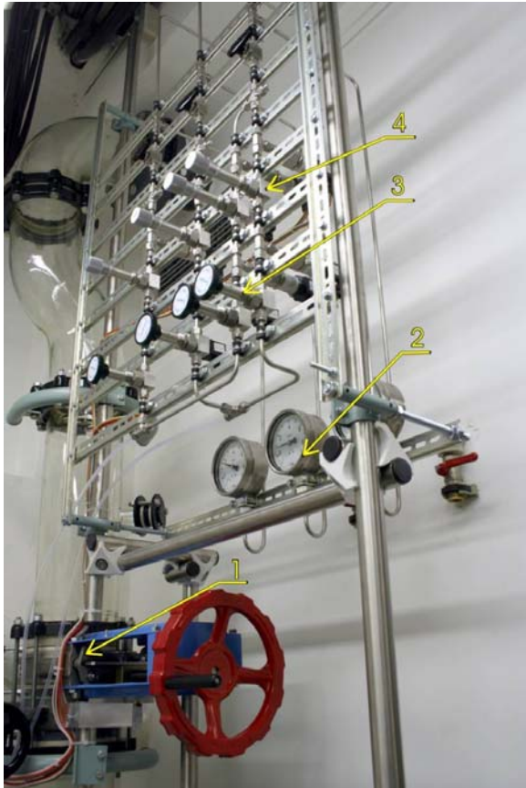
Photo 17. Device details 1 – vacuum shut slide and throttling butterfly valve 2 – pressure meters 3 – control needle valves 4 – measuring needle valves
