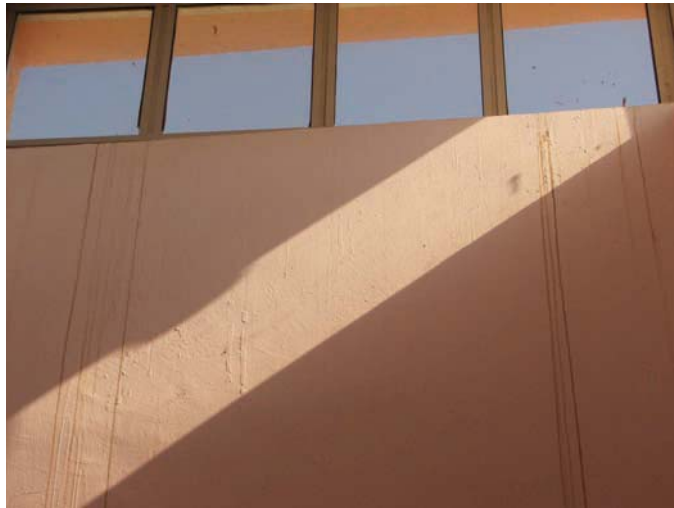
Interior leaks identified during SIGIR site visit.
