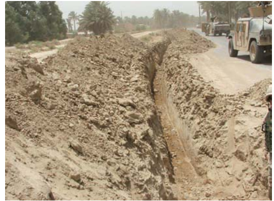
Al Sumelat water pipeline, Baghdad.
