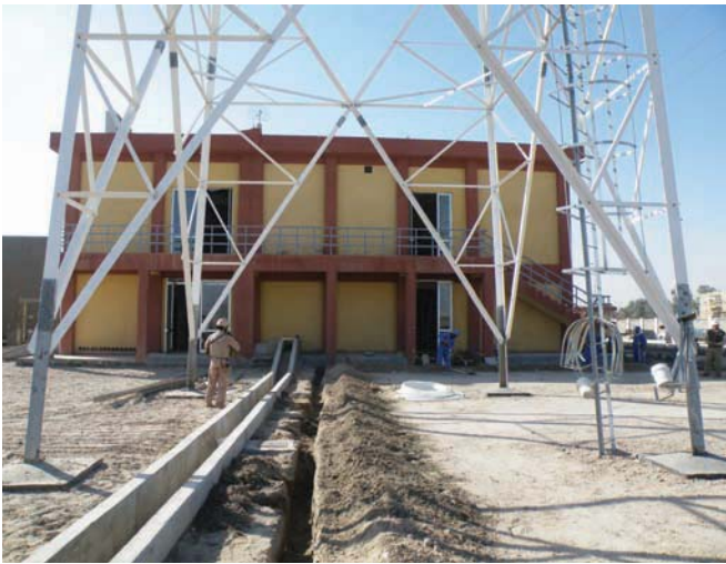
Cable trenches leading into substation building.
