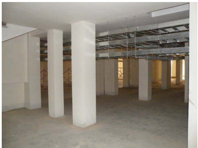
Interior substation ground floor columns and cable trays.
