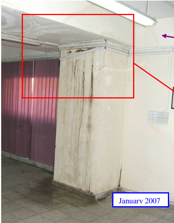
Site Photo 23. Water damage within the ground floor Operations Room from our first site visit
