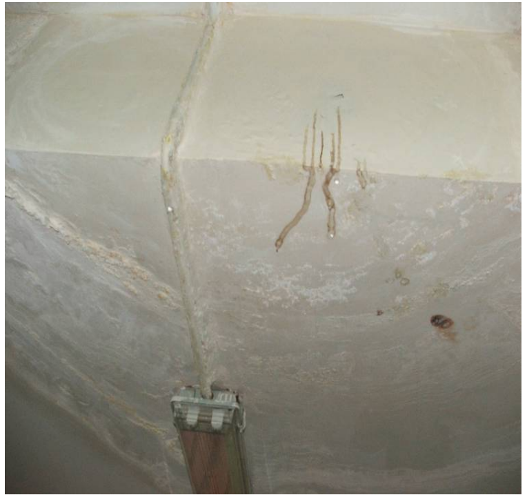
Site Photo 21. Close up view of water damage on ceiling
