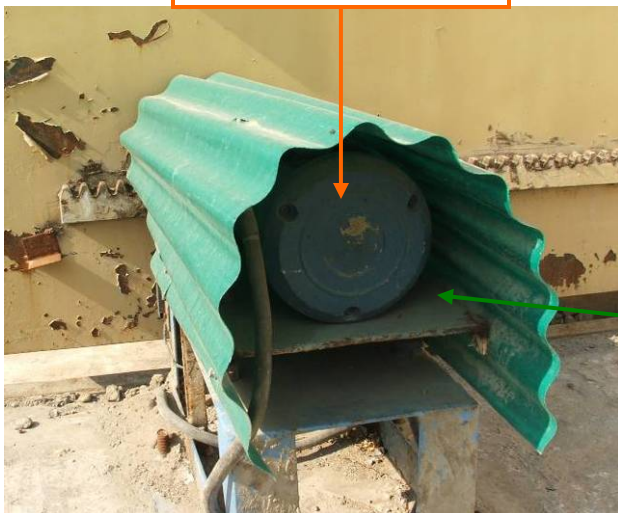
Site Photo 53. Enlargement of Sally Port gate motor
