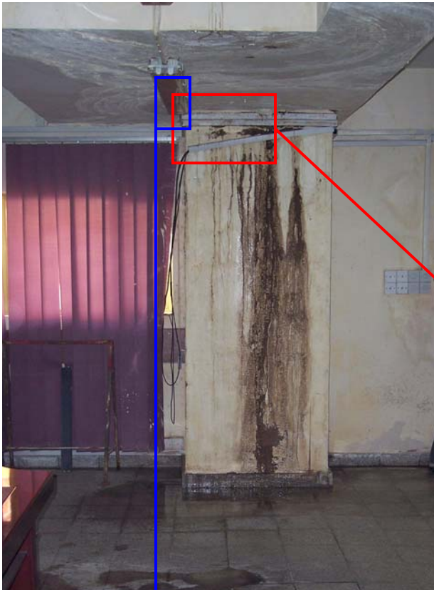
Site Photo 39. Water damage to ground floor Operations Room
