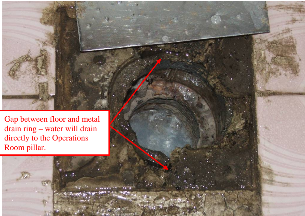
Site Photo 35. Poorly installed floor drain in the first floor bathroom
