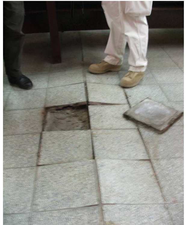
Site Photo 43. Additional view of tile buckling
