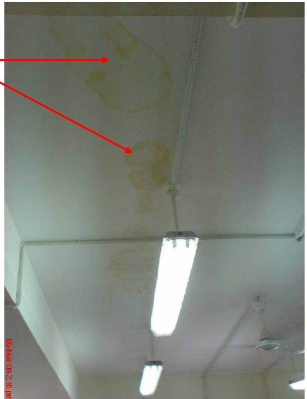
Site Photo 64. Water damage identified in previous QA reports (Photo courtesy of USACE)
