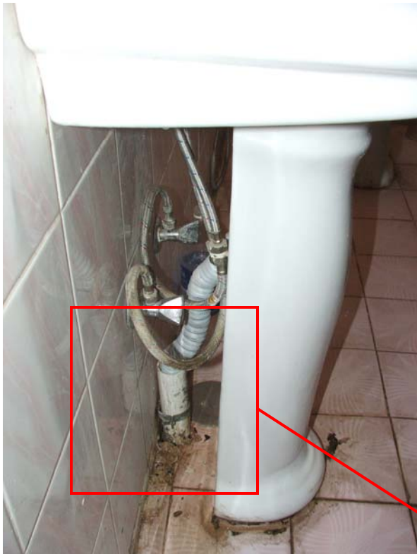
Site Photo 18. Poor installation workmanship (floor not completely waterproofed)
