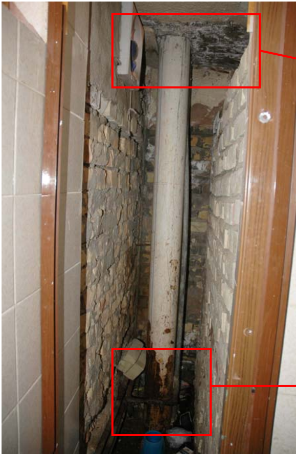
Site Photo 32. Water damage within the first floor bathroom chase
