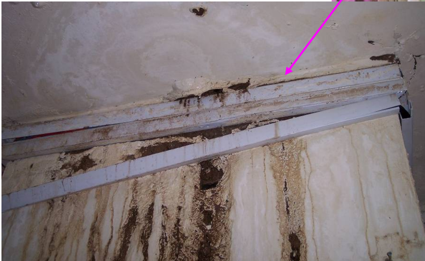
Site Photo 25. Close-up view of water damage
