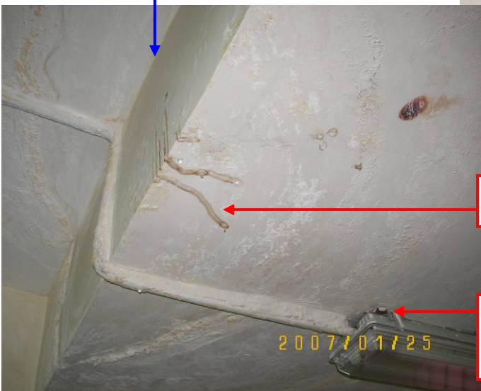
Site Photo 41. Leaking water on the ceiling and open area of light fixture
