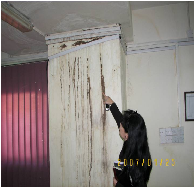
Site Photo 20. Water damage in ground floor Operations Room
