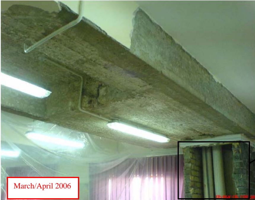
Site Photo 29. Area of water damage to the ground floor Operations Room replaced by the subcontractor in April 2006 (Photo courtesy of the USACE)
