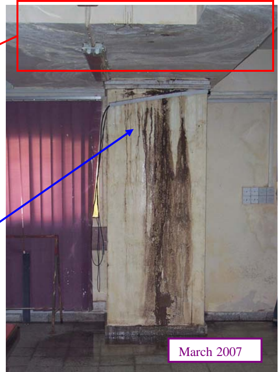
Site Photo 66. Water damage one year later
