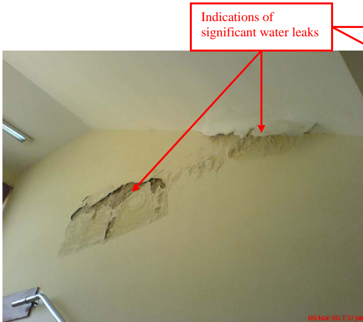
Site Photo 63. Water damage identified in previous QA reports (Photo courtesy of USACE)
