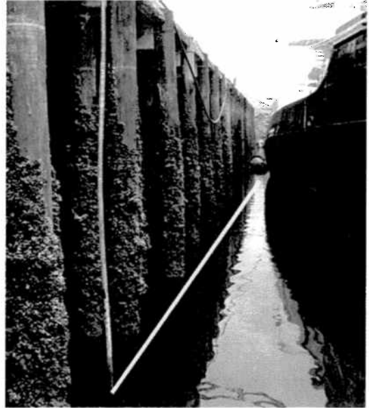
Figure 28 – Missing camels along pier exteriors
