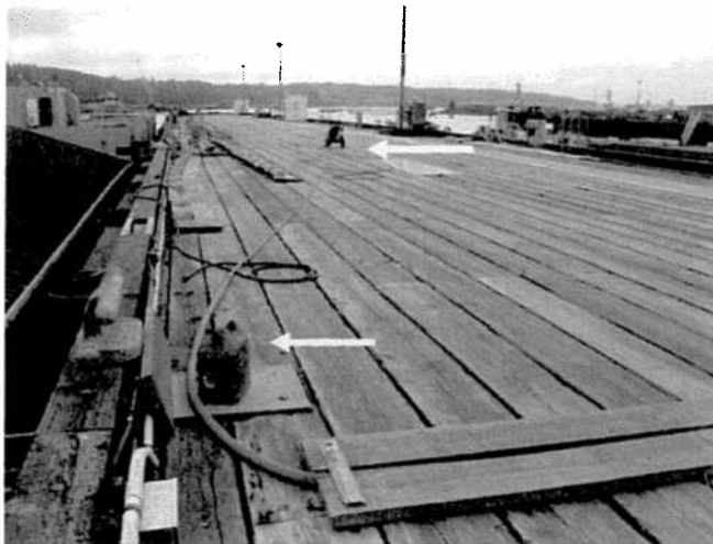
Figure 29 – Temporary utilities on pier deck
