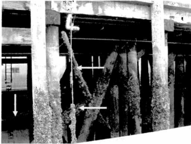
Figure 27 – Debris under Pier Echo
