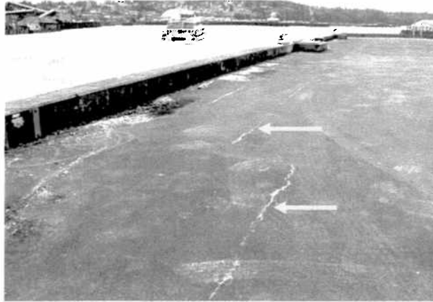
Figure 23 – Concrete surface cracks
