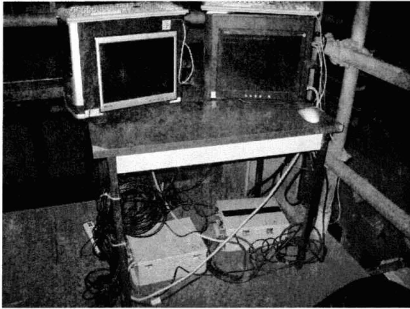
Figure 3-16: Photograph of the NILM location for the 1SA & 3SA Switchboards.
