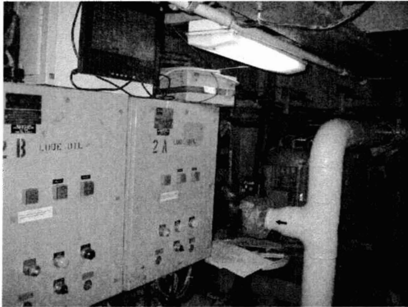
Figure 3-13: NILM Intallation on the 2A LO Pump
