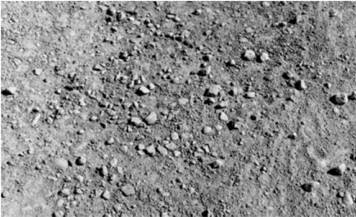
Loose Aggregate, Amber Severity
