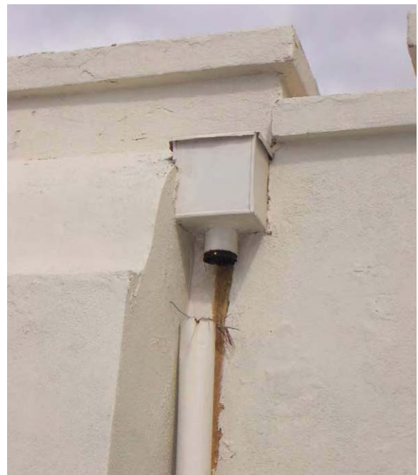
Building 243 – An evaluation of this building would reveal that this is an inappropriate placement for an evaporative cooler.
