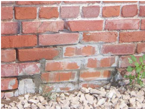
Building 442 – Inappropriate brick and mortar infill.
