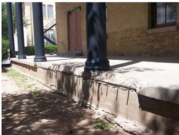
Building 13 – It is not recommended to ignore the crack and the cause for the damaged concrete, allowing for further deterioration of the concrete material.
