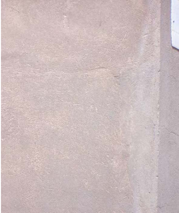
Building 19 – Small hairline cracks usually are not serious and may be sealed with a thin slurry coat consisting of the finish coat ingredients.
