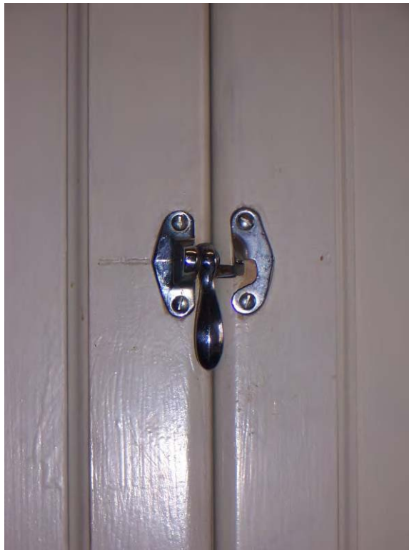
Building 114 – Cabinet door lockset.
