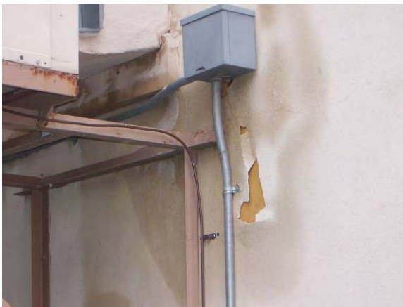
Building 243 – Here water damage is causing paint deterioration on a stucco wall. Remove damaged or deteriorated paint only to the next sound layer using the gentlest method possible (e.g., hand-scraping) prior to repainting.
