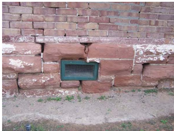
Building 128 – It is important to keep moisture away from sandstone foundations. Note areas where there is missing mortar or loose stones.
