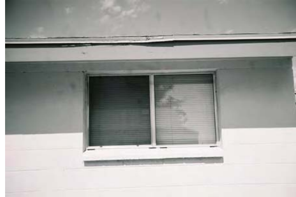
Building 9414 – It is recommended to replace an entire window that is too deteriorated to repair using the same design details such as number of lights, panels and hardware. If using the same kind of material is not technically feasible then a compatible substitute material may be considered. Above is an inappropriate replacement metal slider window. The original was a four-pane metal awning window.
