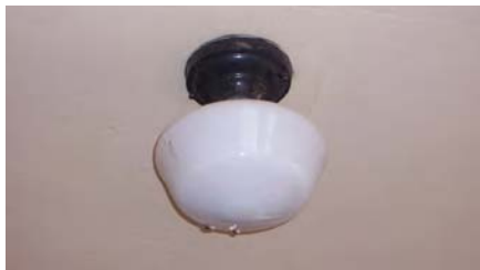
Building 515 – Good example of interior light fixture.
