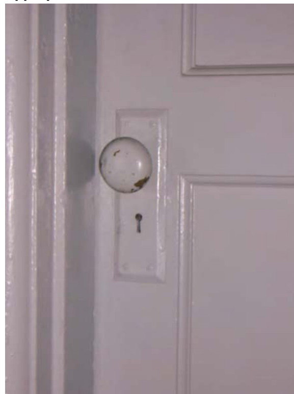
Building 114 – Appropriate interior knob and lockset.
