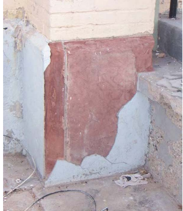
Building 21 – A thin layer of stucco is used over some sandstone features like foundations found at Fort Bliss. Evaluate the condition of the stucco and determine the appropriate repair method needed to protect and maintain the sandstone feature. Remember patching should be in-kind to the existing material.
