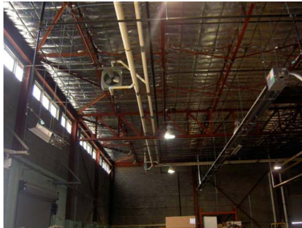
Figure 30. Interior of portions of Bldg. 2592 are very dark, even with artificial lighting.
