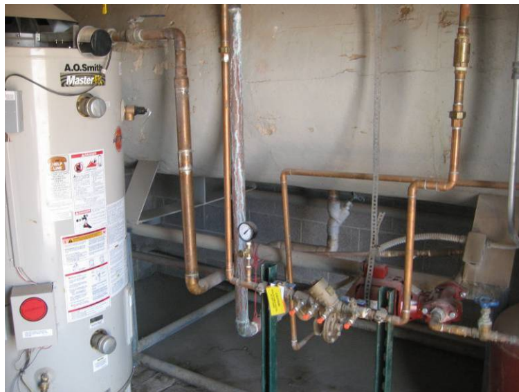
Figure 28. Uninsulated hot water piping, Bldg. 5041.
