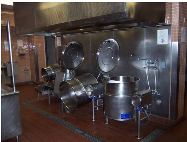
Figure 17. Cooking equipment under exhaust hood.
