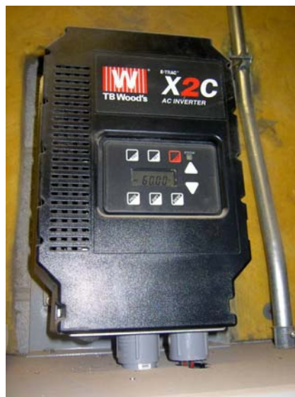
Figure 13. AHU-3 inverter in Bldg. 11293 continually operates at 60 Hz.
