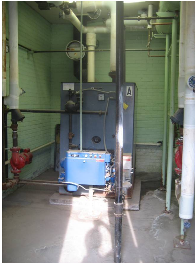
Figure 27. Boiler in Bldg. 622.
