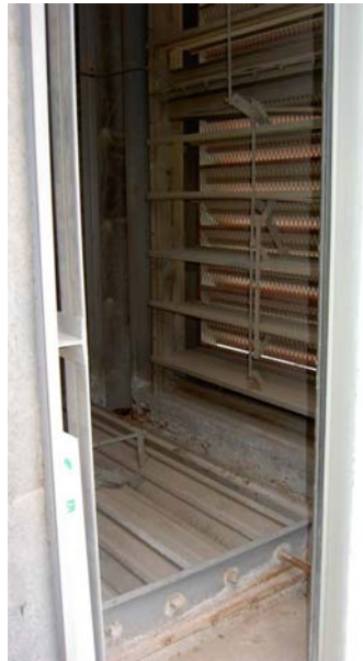
Figure 14. Bldg. 2457, Dining Hall, OA and RA dampers not operating correctly.
