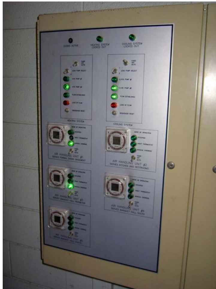
Figure 15. Existing control panel in the Centennial Club mechanical room, Bldg. 11199.
