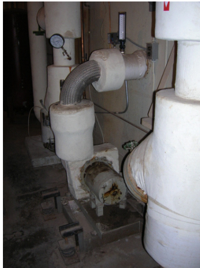
Figure A-3. Chilled Water Pump
