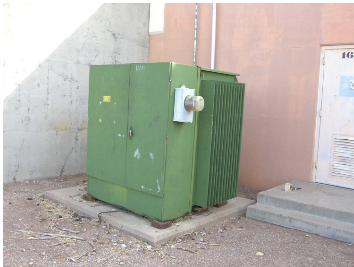
Figure A-8. Commercial Power Transformer
