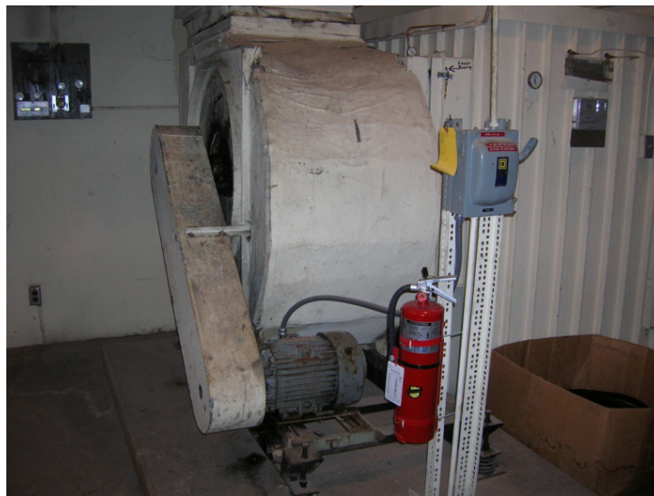
Figure A-4. Air Handler
