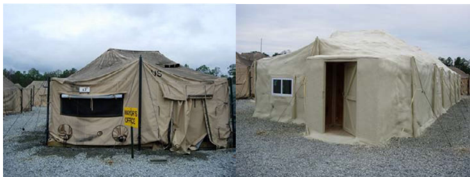
Figure: Tent before Application of Foam Insulation and Tent after Application of Foam Insulation
