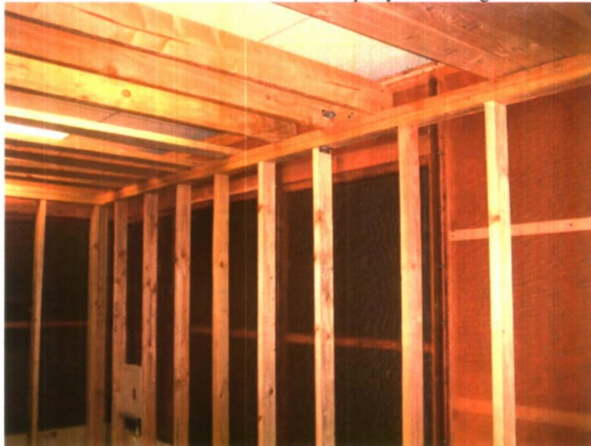
Fig. 9: Ferrite Tile Support Structure inside EMC Screen Room: 2" × 6" Ceiling Joists
