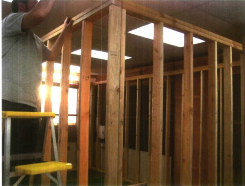
Fig. 8: Ferrite Tile Support Structure inside EMC Screen Room
