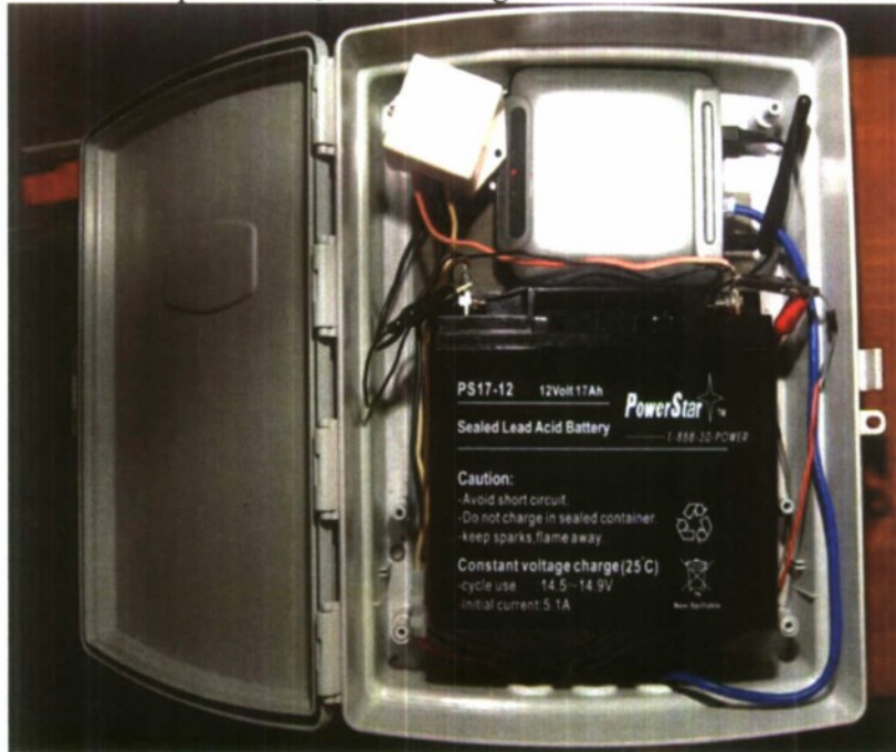
Figure 12 - Access Point, charge controller, and battery in weatherproof casing
