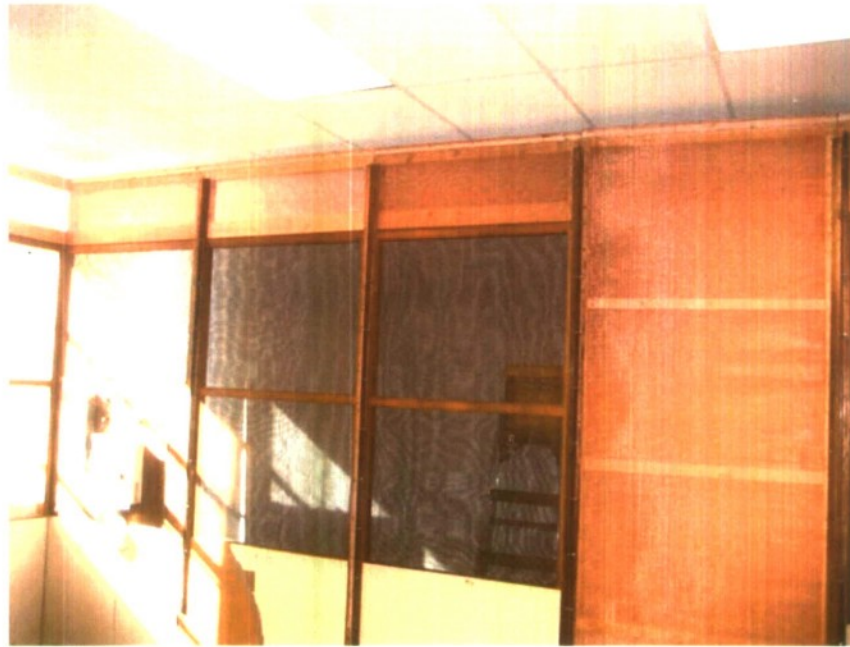
Fig. 6: EMC Screen Room Expansion: Note new panel on right, 1ft height extension panels
