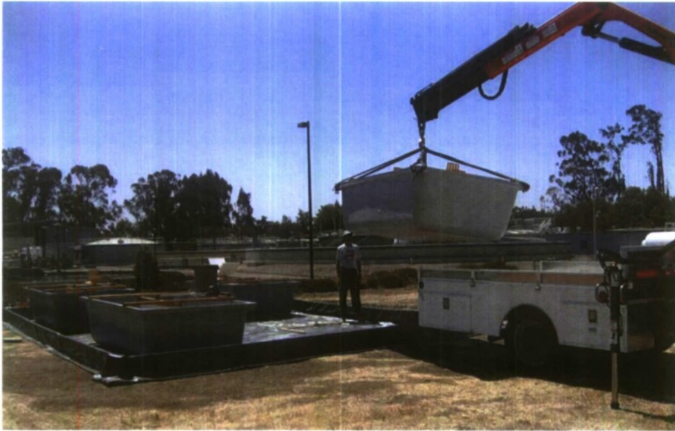
Figure 2-3. Placement of HRPs in secondary containment using knuckle boom provided by the SLO WRF.
