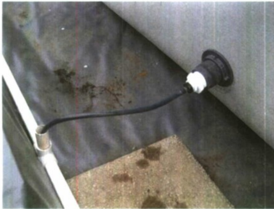
Figure 2-5. HRP effluent tank adaptor, tubing, and piping.
