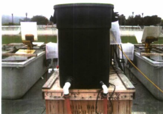
Figure 2-9. Influent constant-head feed tank with inflow and outflow piping back to the clarifier.
