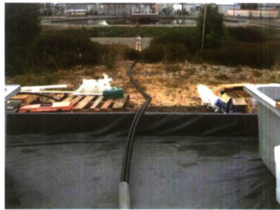
Figure 2-8. Influent tubing from the clarifier crossing the secondary containment wall.
