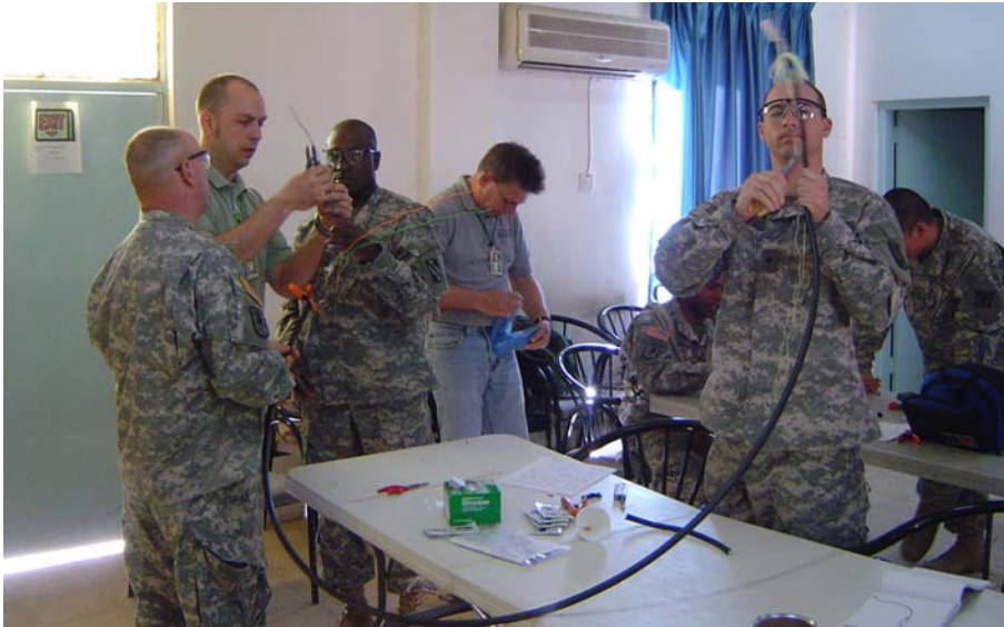
SGT Frank Ferguson, SSG Lonnie Colvin, and SPC Justin Rubio from the 842nd Signal Company conduct fiber training with Brad Smoczyk and Paul Johnson from the Anteon engineering and installation team.
