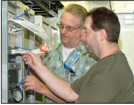
Ken Stackhouse, left, and Stephen Koval, configure an Internet interface router rack in the Auxiliary Communications Shelter at Tobyhanna Army Depot. The shelter supports the homeland defense Ballistic Missile Defense System. Stackhouse and Koval are electronics technicians in the depot's Production Engineering Directorate.
