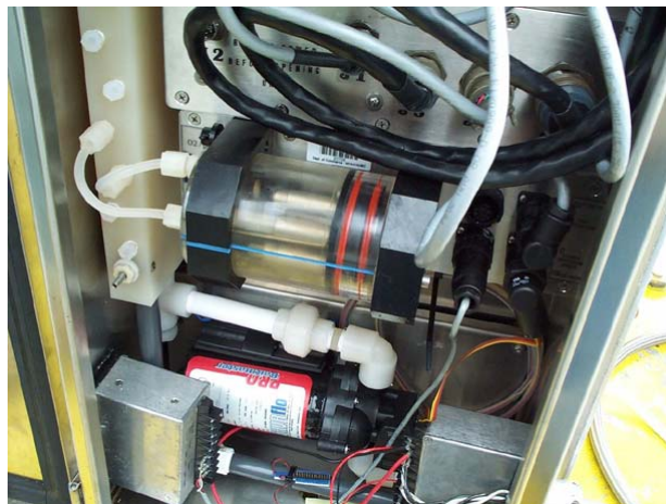
Fig. 2. Sensors in OSM enclosure
