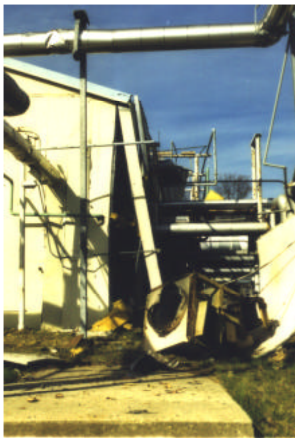
FIGURE 9. DAMAGE TO NEARBY EQUIPMENT BUILDING
