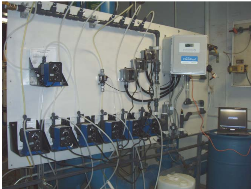
Figure 2. Smart monitoring and control system.
