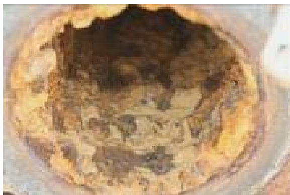
Figure 11. Corroded hot water supply line.
