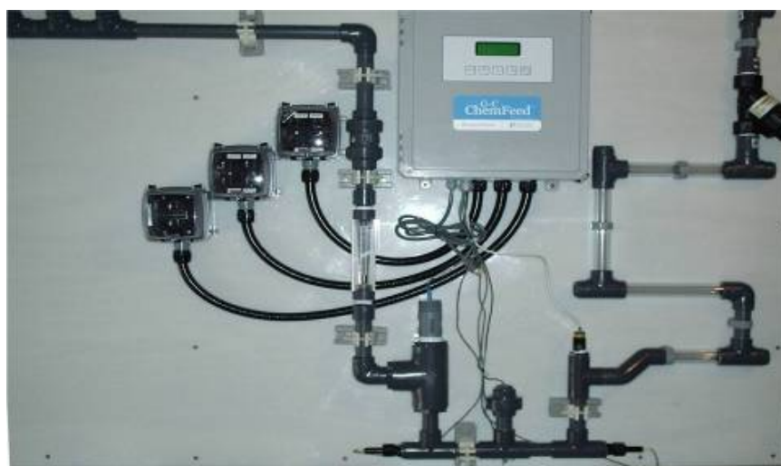
Figure 6. Cooling system controller.
