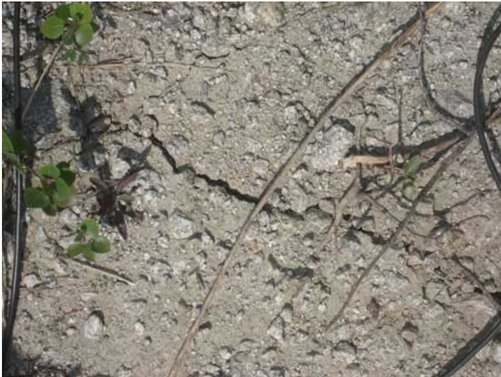
Figure 76. Crack from Shot 4 observed while walking around the borehole.
