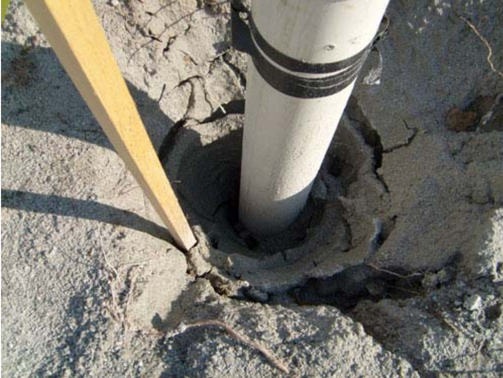
Figure 100. Grout collapsed around PVC pipe in a cross-hole tomography bore hole.
