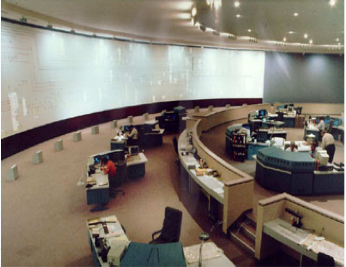
Figure 2.10: SCADA master control station [6]
