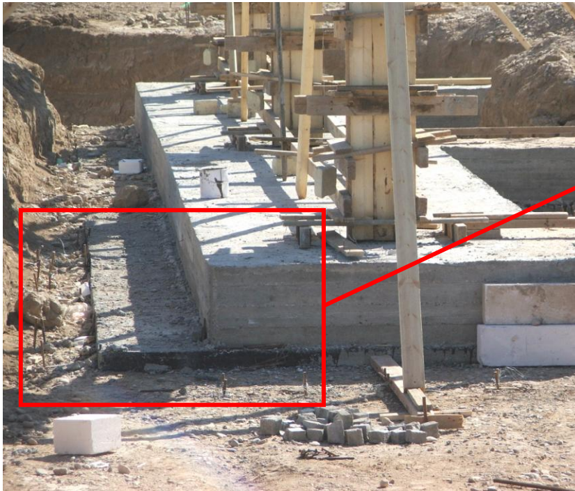
Site Photo 19. Examples of protruding reinforcement bar
