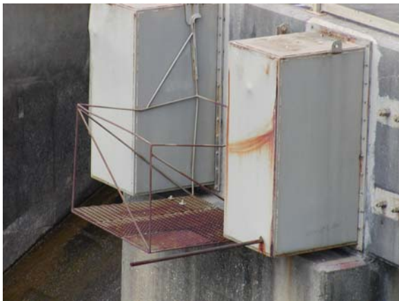
Figure 8. Anchor rod covers and a failed anchor rod that shot through the cover.
