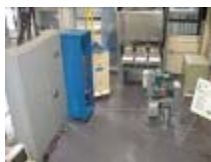
Electrical Power Architecture Lab
