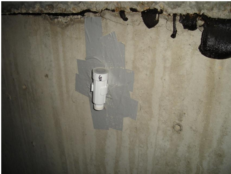
Figure 15. A HOBO Pro v2 temperature/humidity sensor placed on the wall of a septic tank.
