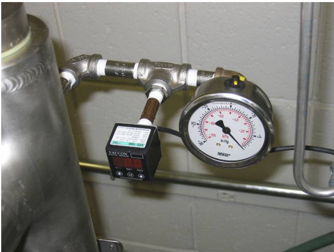
Figure 21. Relocated Digital and Mechanical Vacuum Gauges
