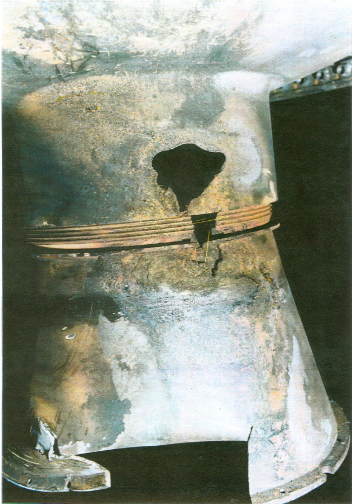
Figure 5b. Nozzle Exit Cone Assembly Burnthrough
