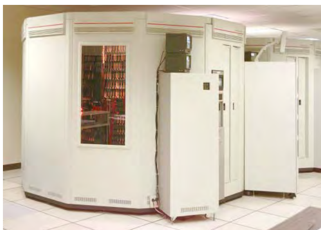
StorageTek 9310 tape silos
