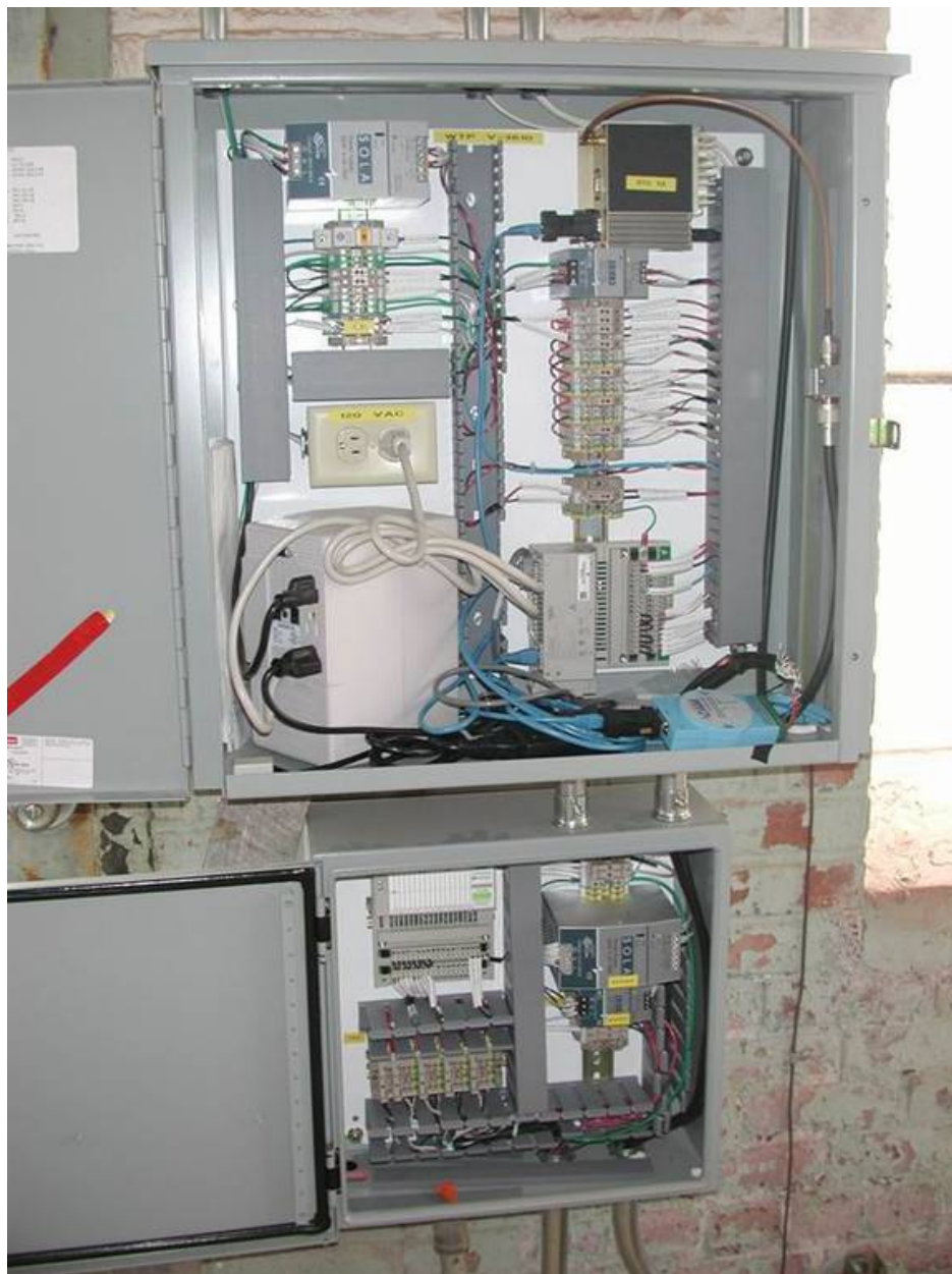
Figure 11. Typical SCADA box at Fort Bragg.
