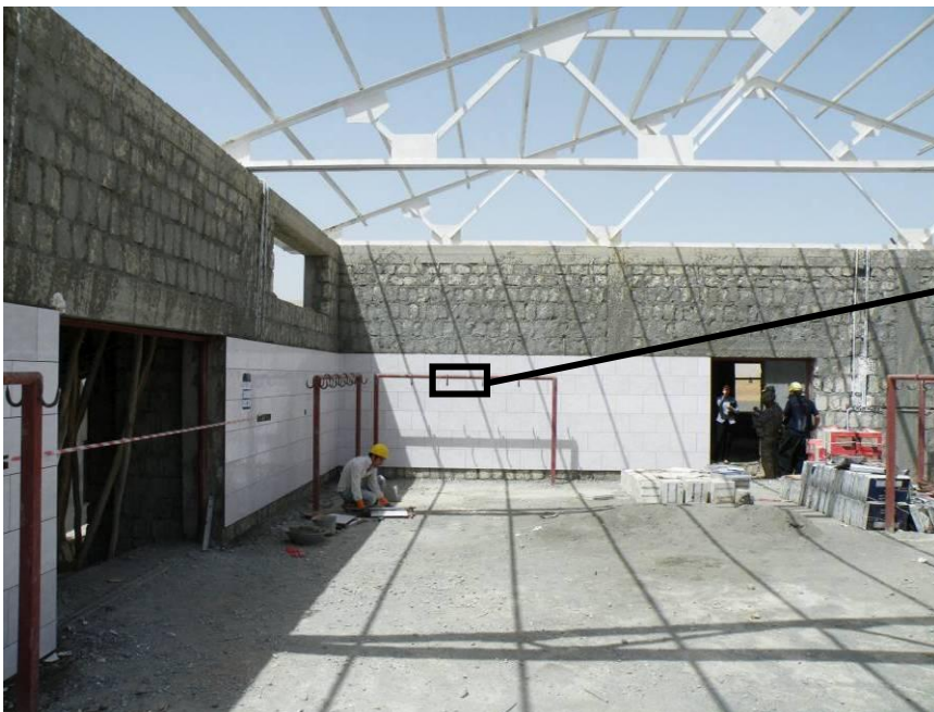
Site Photo 21. Exposed meat support hooks located throughout facility
