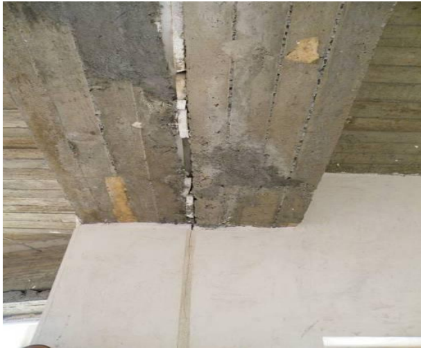
Site Photo 16. Correctly designed/placed ceiling beam expansion joints
