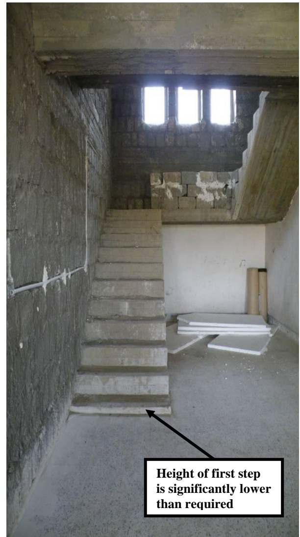
Site Photo 20. Bottom step poses tripping hazard
