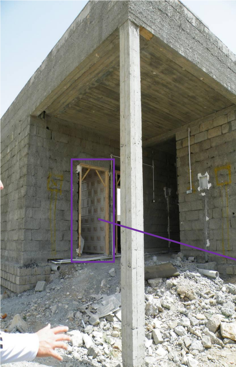
Site Photo 7. Concrete floor and roof slabs poured for the guard house
