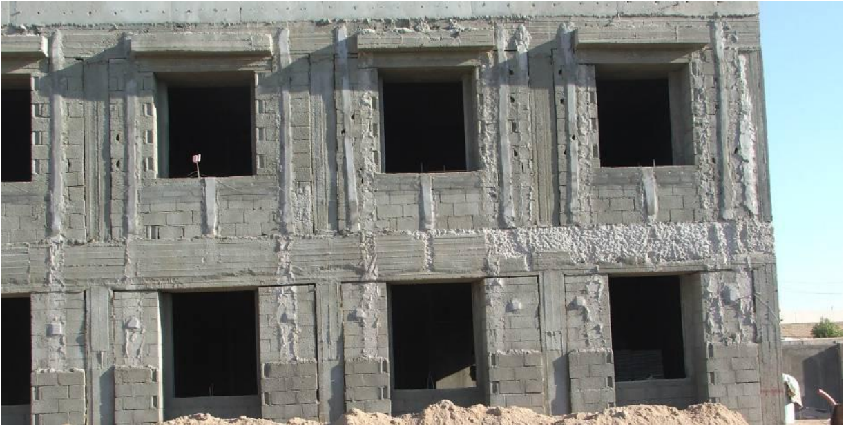
Site Photo 24. Poor structural concrete work
