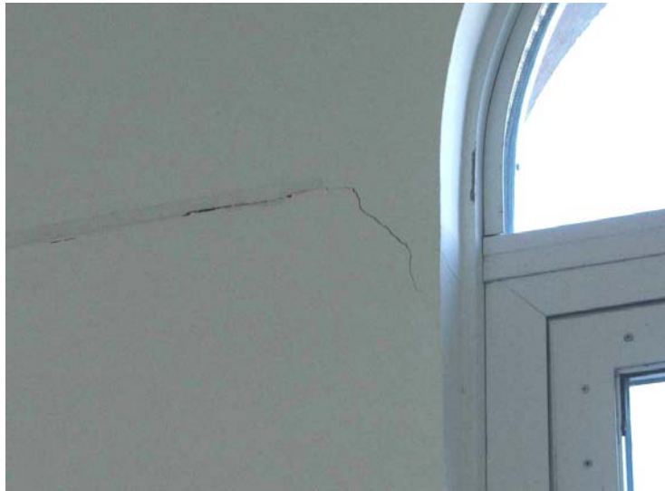
Site Photo 18. Poorly constructed control joints
