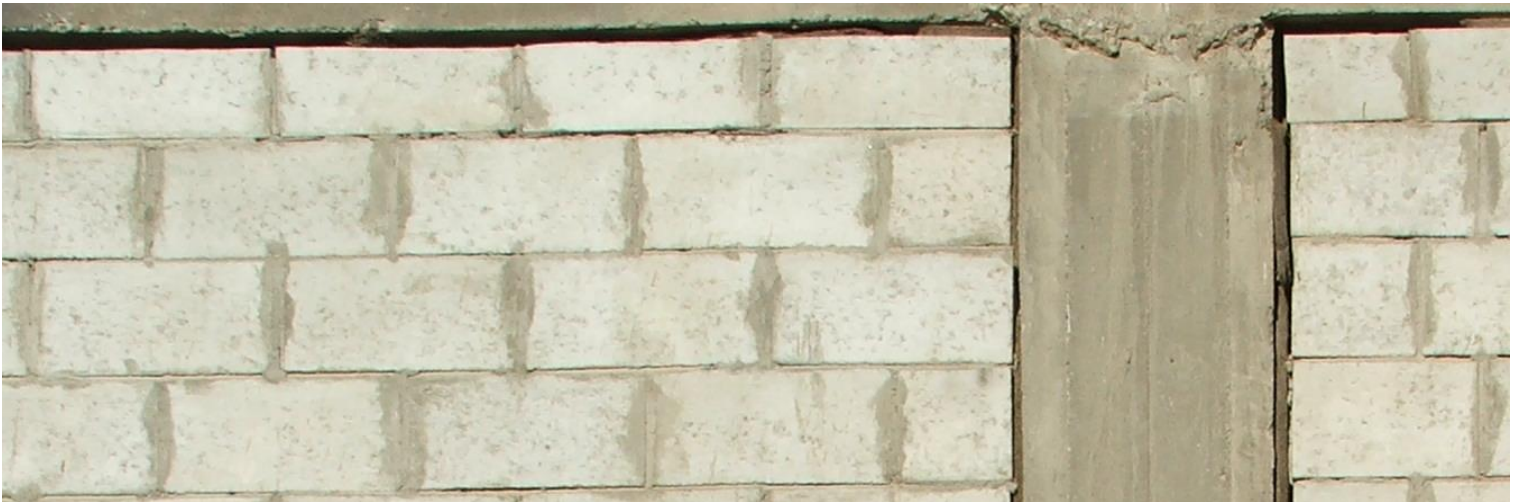
Site Photo 25. Poor block in-fill work
