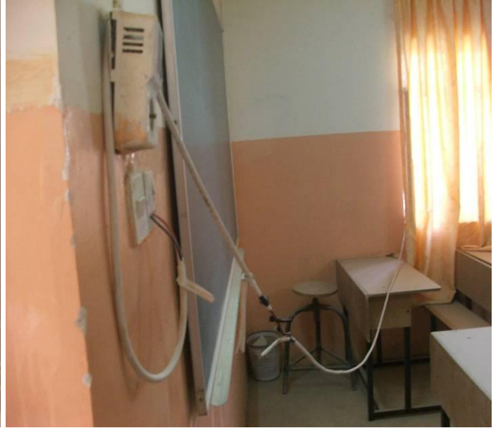
Site Photo 36. Improper electrical connection (Al Mualameen)
