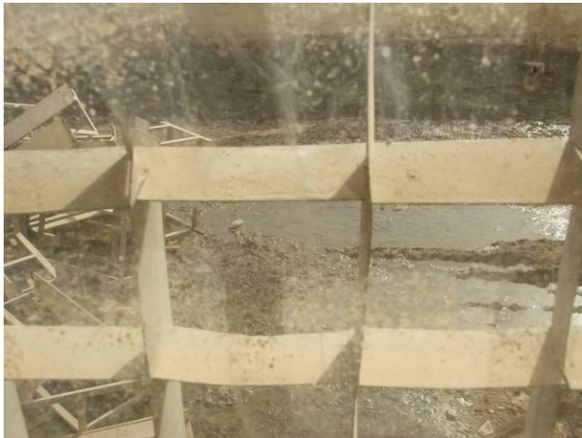
Site Photo 41. Exterior debris (Al Faoo)
