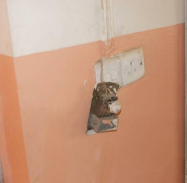
Site Photo 35. Poor electrical installation (Al Mualameen)
