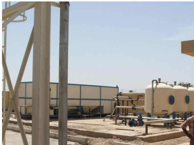
Site Photo 8. Water compact unit
