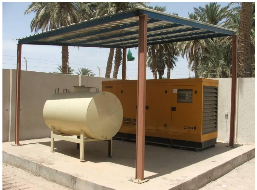
Site Photo 7. Sunshade for the generator and the fuel tank.
