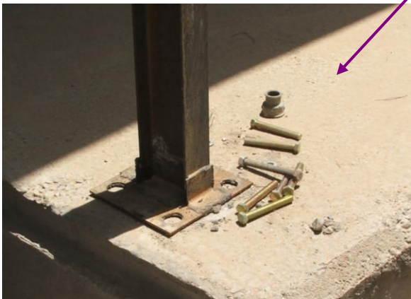
Site Photo 13. Unbolted sunshade post
