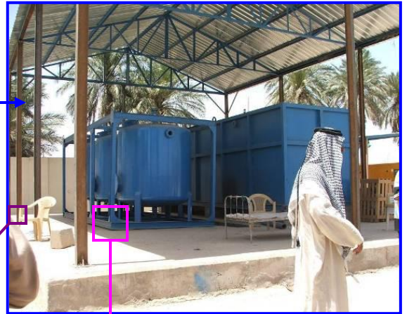
Site Photo 12. Water compact unit sunshade
