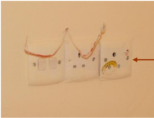
Site Photo 9. Inadequate electrical work
