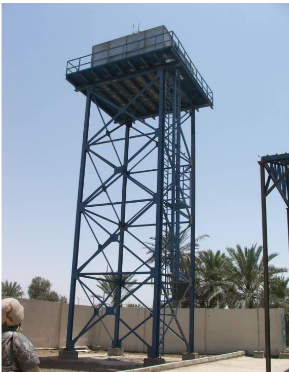
Site Photo 6. Elevated reservoir storage.
