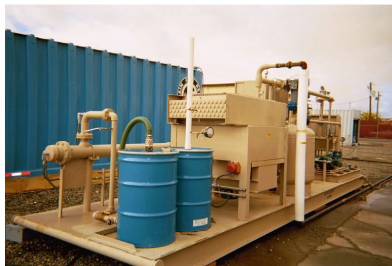
(c) Vapor-Extraction Treatment System
