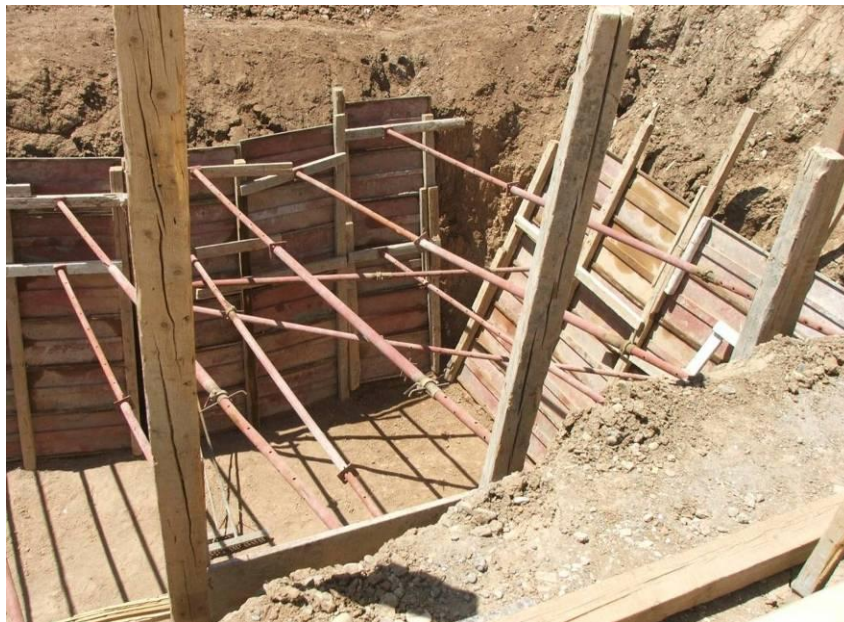
Site Photo 15. Improperly braced shoring for septic tank construction.
