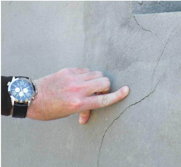
Site Photo 14. Cracking of the surface coating on the block walls and columns
