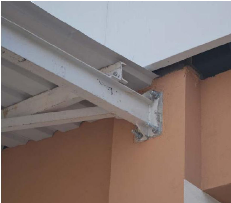
Site Photo 16. Corrective fix to the perimeter awning (Courtesy of USACE)
