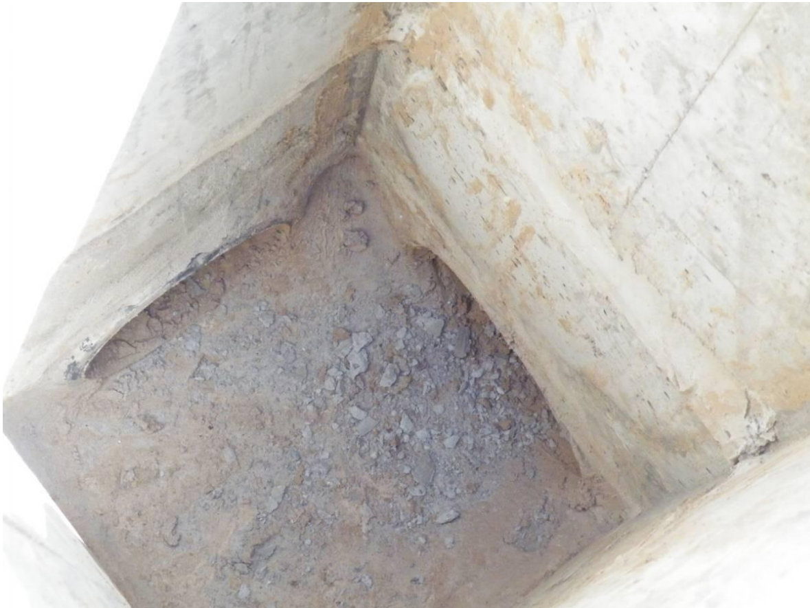
Site Photo 11. Sanitary sewer manhole with debris and no access steps
