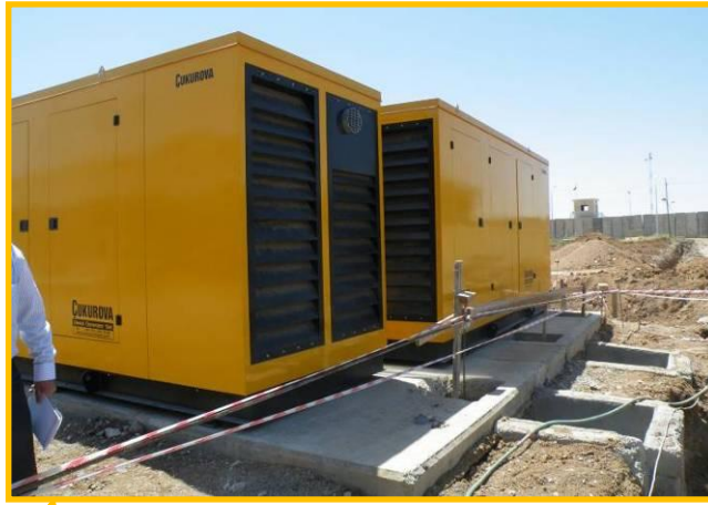
Site Photo 2. Generator pad with generator
