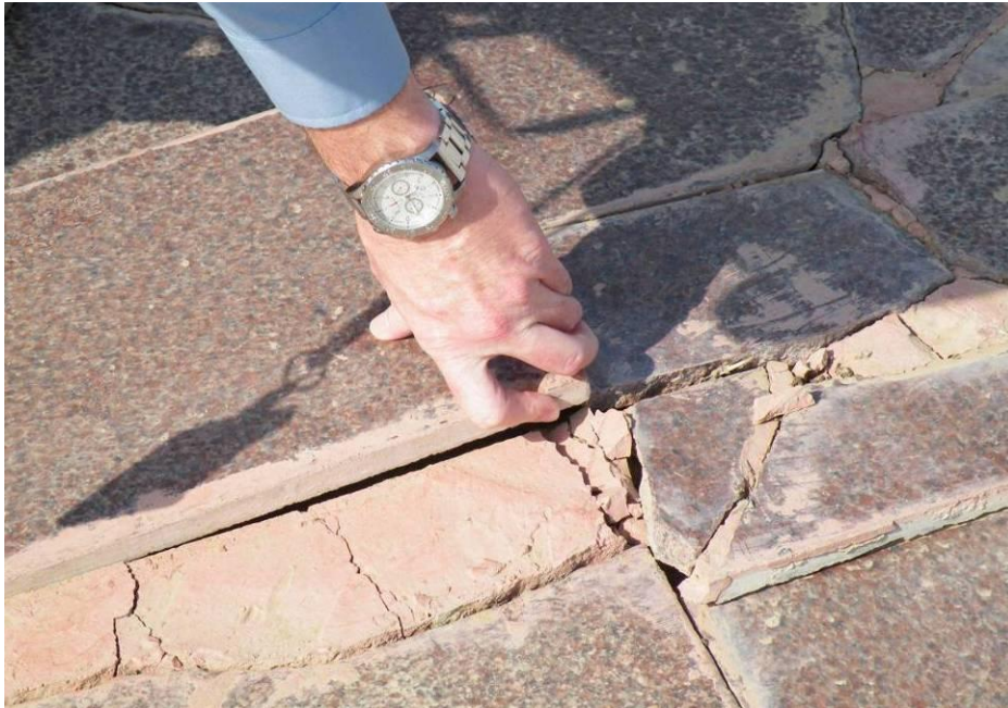
Site Photo 6. Cracked and raised concrete tiles
