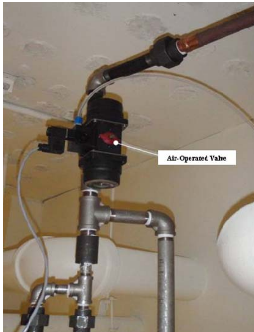
Figure 14. Exhaust System's Pneumatic Ball Valve
