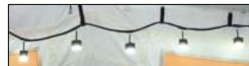
Shelter LED Lighting with Ambience
