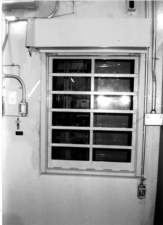
Observation window in concrete wall showing security grille and fire shutter
