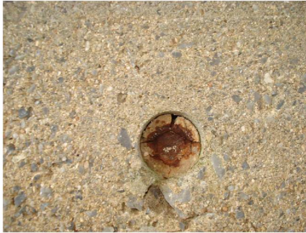
Figure 13. Typical steel within a delaminated "plug."
