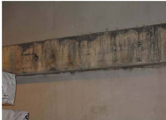
Figure 1c. Closer view of beams "A" before treatment
