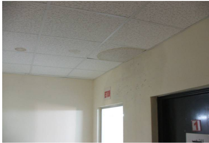
Site Photo 28. Example of water leakage
