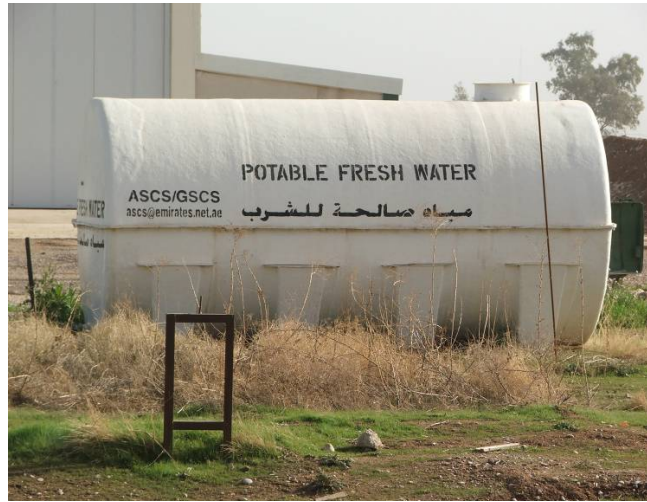
Site Photo 31. Potable water supply
