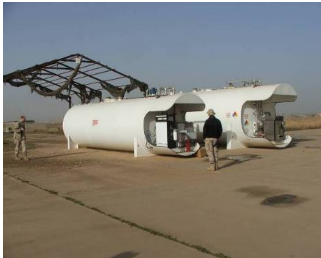
Site Photo 32. Two fuel tanks
