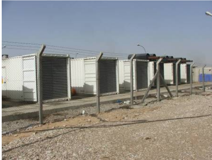
Site Photo 12. Eight 1MW electrical generators
