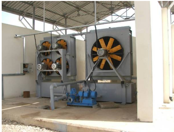
Site Photo 31. Generator building cooling system
