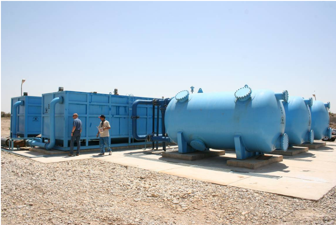
Photo 5. Drinking water treatment plant.
