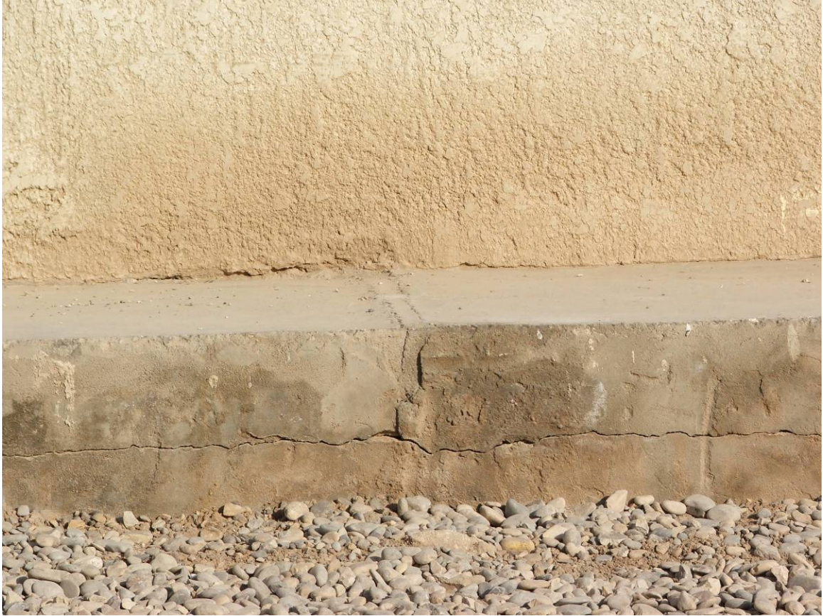
Site Photo 23. East barracks horizontal foundation fracture.
