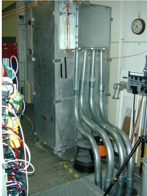
Figure 62. Data-cable conduits and Hoffman box covering patch panel
