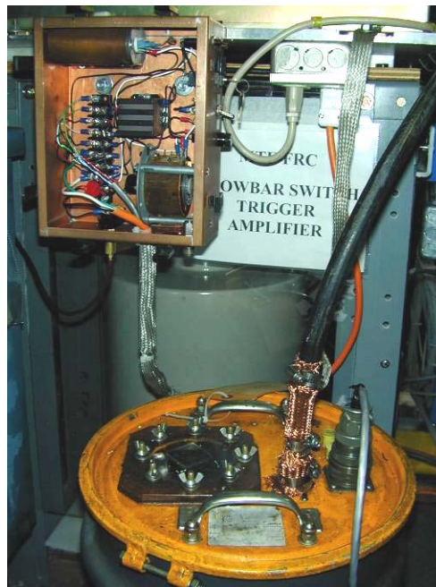
Figure 72. Remotely operated controller (upper left) fabricated for Crowbar Switch's UV power supply
