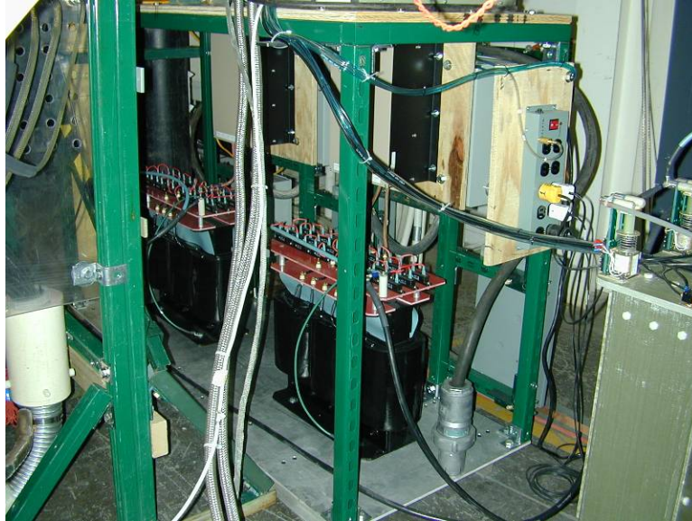
Figure 35. Upper and Lower Cusp bank power-supply stand
