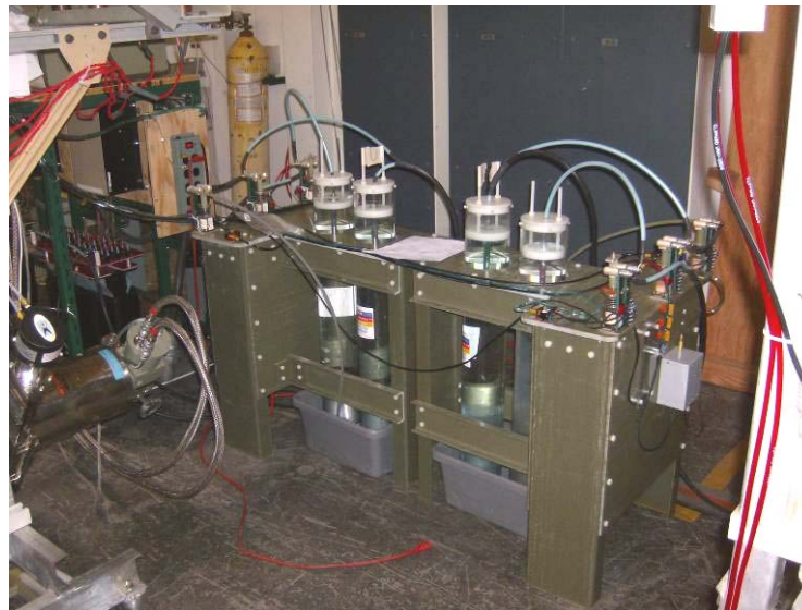
Figure 36. Resistor stands for Upper and Lower Cusp banks, between power-supply stand and Cusp banks
