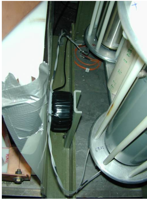
Figure 27. New 1:1, dual-secondary isolation transformer for Bias bank ignitron trigger unit With this transformer, the original trigger unit was now able to trigger both ignitrons, and there were no issues with jitter. The pulses provided to both ignitrons were monitored a few times before the bank was actually charged and triggered, Figure 28 shows the observed waveforms.
