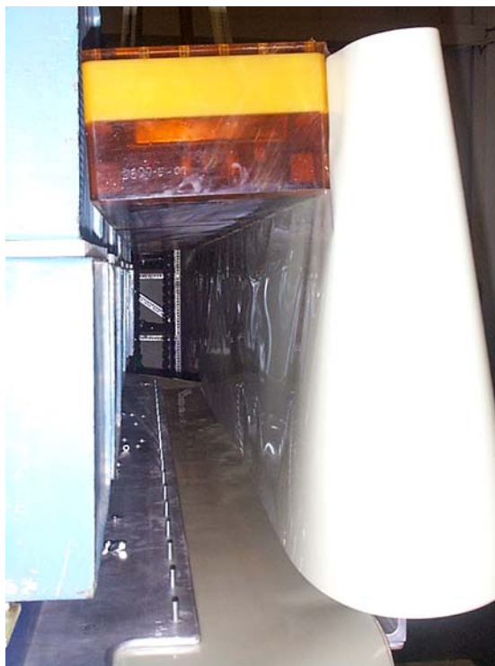
Figure C3. Integral nature of FRCHX Main bank and Crowbar switch bus work
