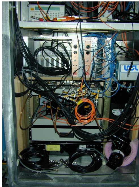
Figure 55. Detectors and RF demodulator circuits for four-chord interferometer Once the interferometer-optics table was in place, it was discovered that one of the all-thread rods running through the Cusp and Theta coil assembly was blocking the path of the fourth chord. The fourth chord is used primarily to correct for the heating in the quartz tube during a shot, but in order to serve this purpose its path must lie outside the plasma in the tube. (See
