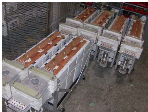
Figure 96. T2-mF Guide/Mirror bank modules, in high bay
