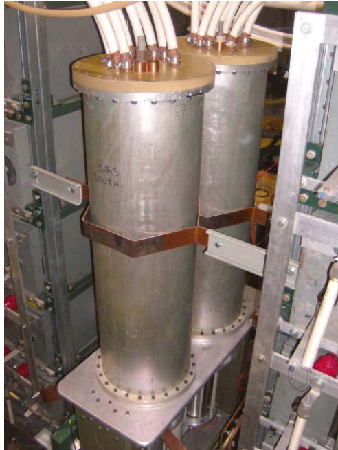
Figure 39. Inductor housings on Bias bank stand
