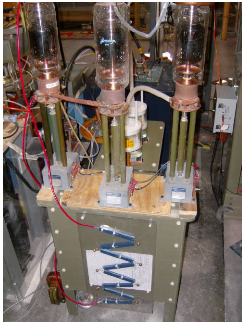
Figure 7. Jennings switches and diode stack on PI bank resistor stand
