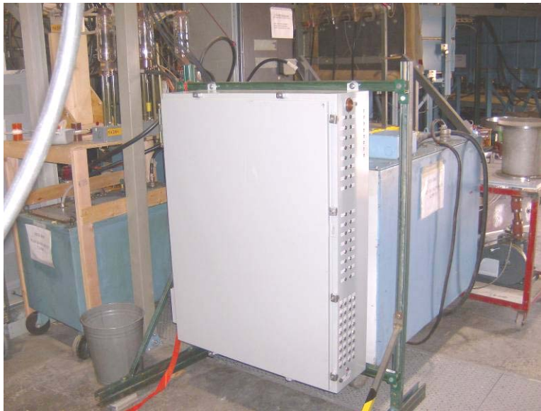
Figure 67. cFP controller, next to Main bank power supply
