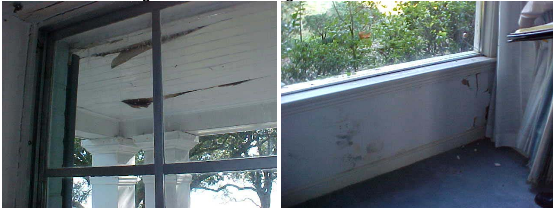
Figures 4 and 5. Damage to Beachfront Homes
