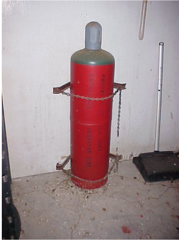
Photograph 23: Acetylene tank in Building T-13.
