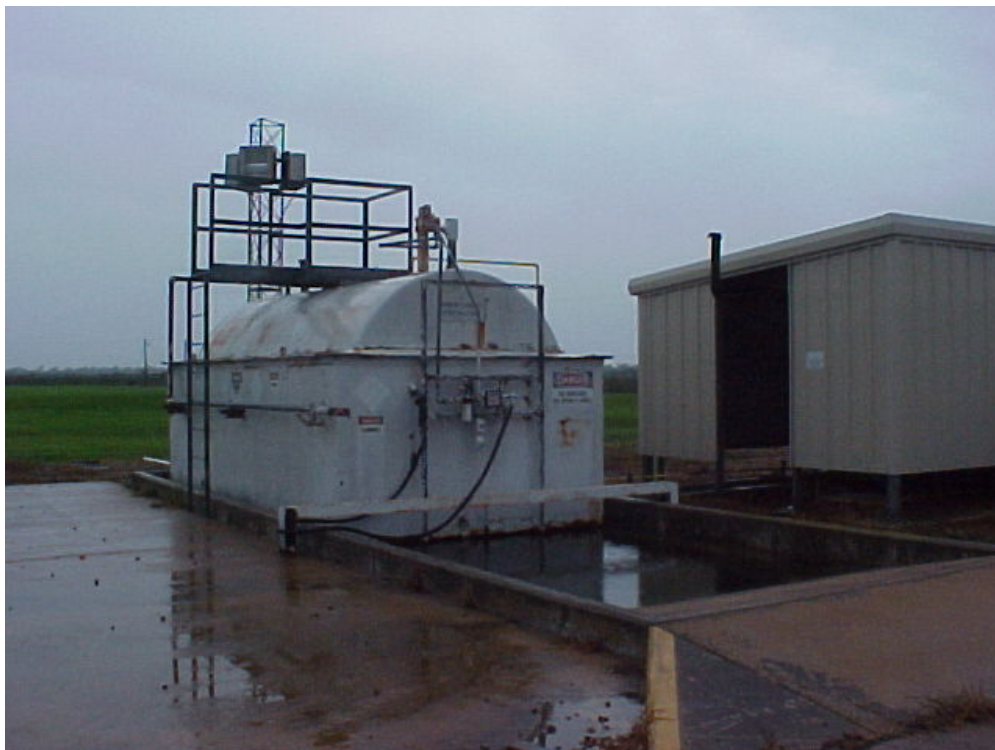
Photograph 2: A fuel line from the AST goes into the adjacent shed where the generator is located.
