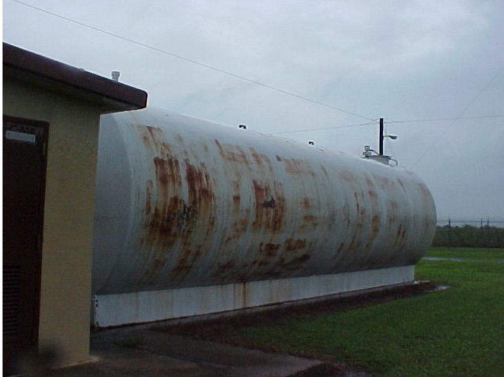
Photograph 9: The water tank is showing corrosion from the Gulf's salt water.
