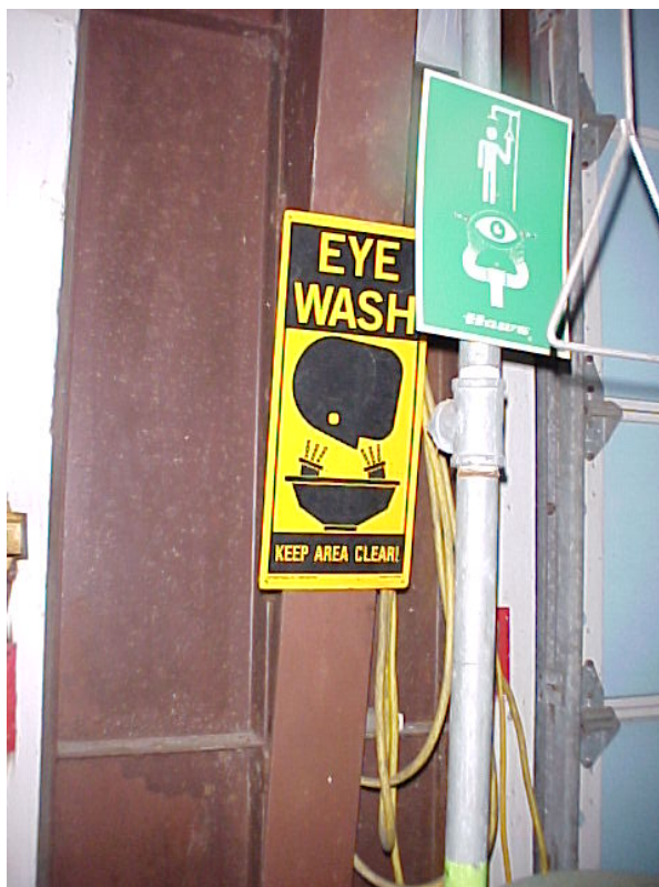
Photograph 27: Eye Wash Station in Building T-13
