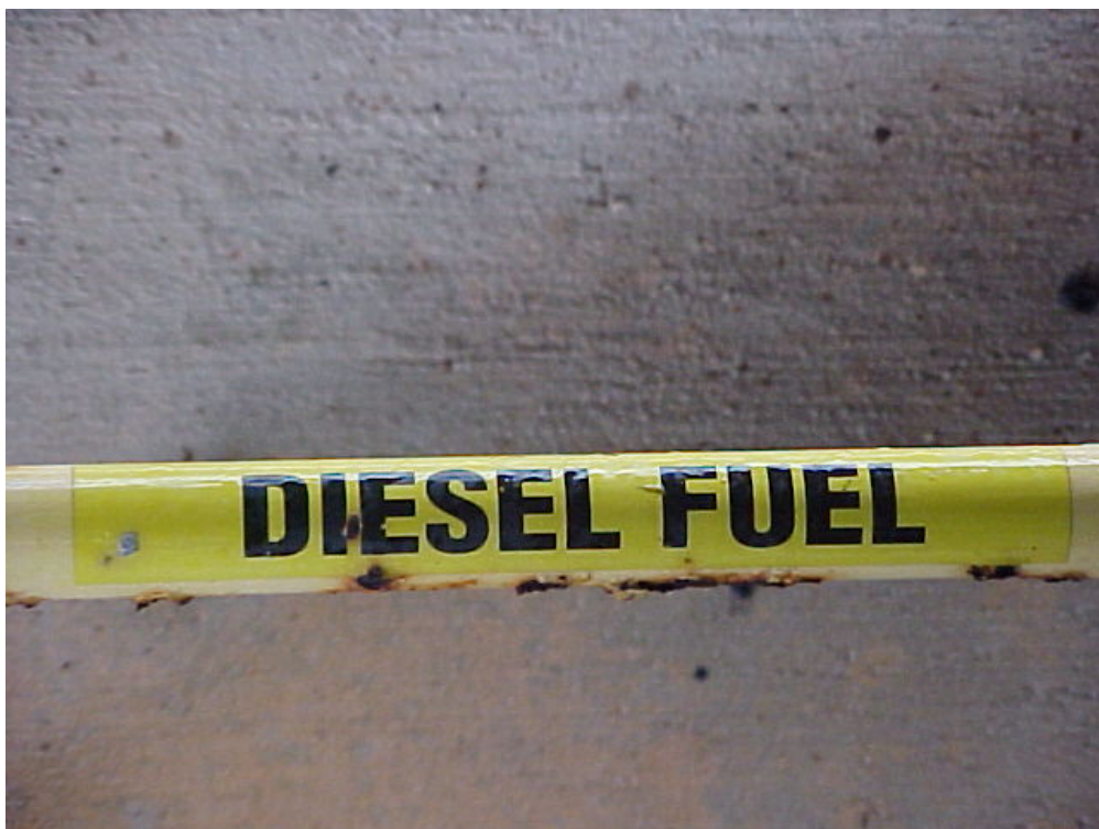
Photograph 4: Lettering on the fuel line at the generator site.
