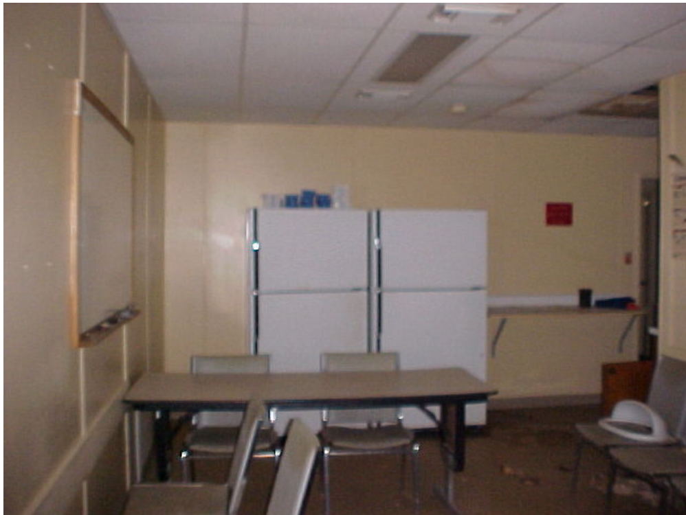
Photograph 40: Break room, furniture, and refrigerators left behind in Operations Building.
