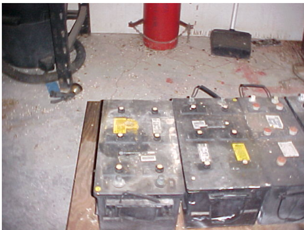
Photograph 26: Batteries stored in Building T-13.
