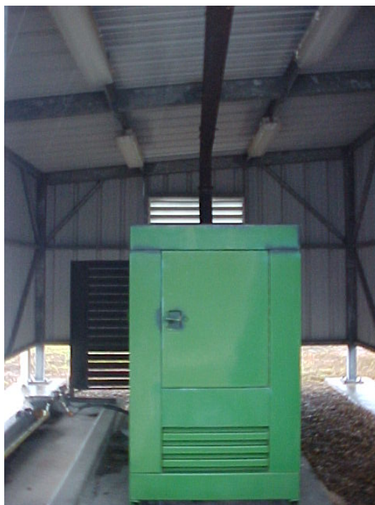
Photograph 5: Generator in the shed. No leakage was observed.
