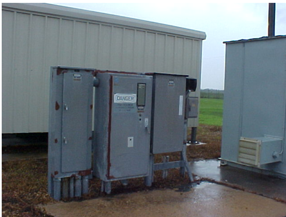
Photograph 6: Transformers at the Matagorda TARS site.
