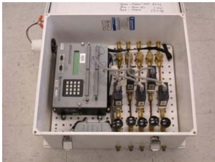
Figure D-3. Datalogger and Mass Flow Regulators.
