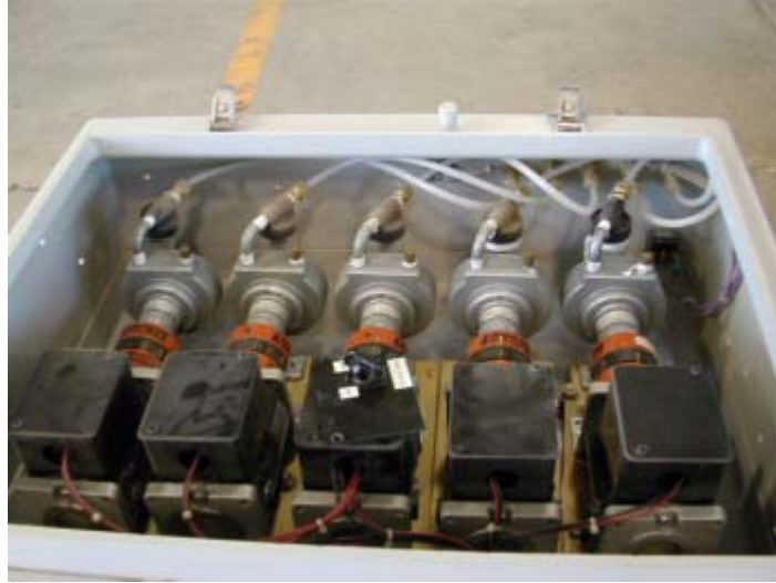
Figure D-4. Vacuum Pumps.
