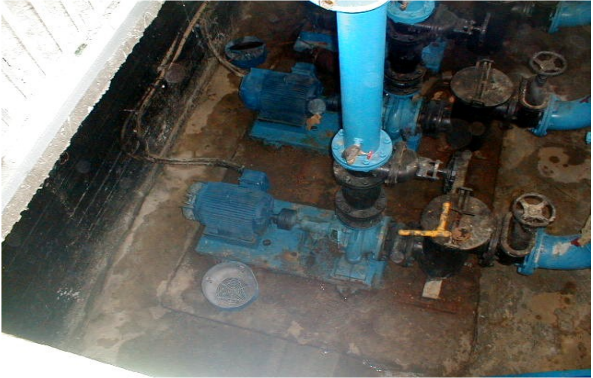
Photo 3. Al Hillah Olympic Swimming Pool Pumps
