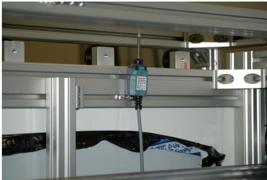
Figure 60: Observatory Internal Safety Switch ( photo credit: Pier-Tech, Inc. 2007 )
