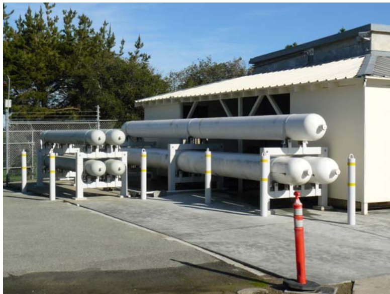
Figure 42. Air farm at NPS rocket propulsion lab
